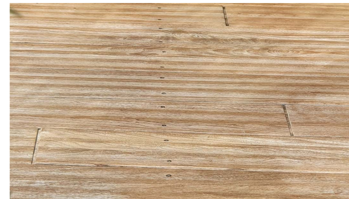
Weathered deck made from thermally treated ash after de-graying with DeckDegrayer.
